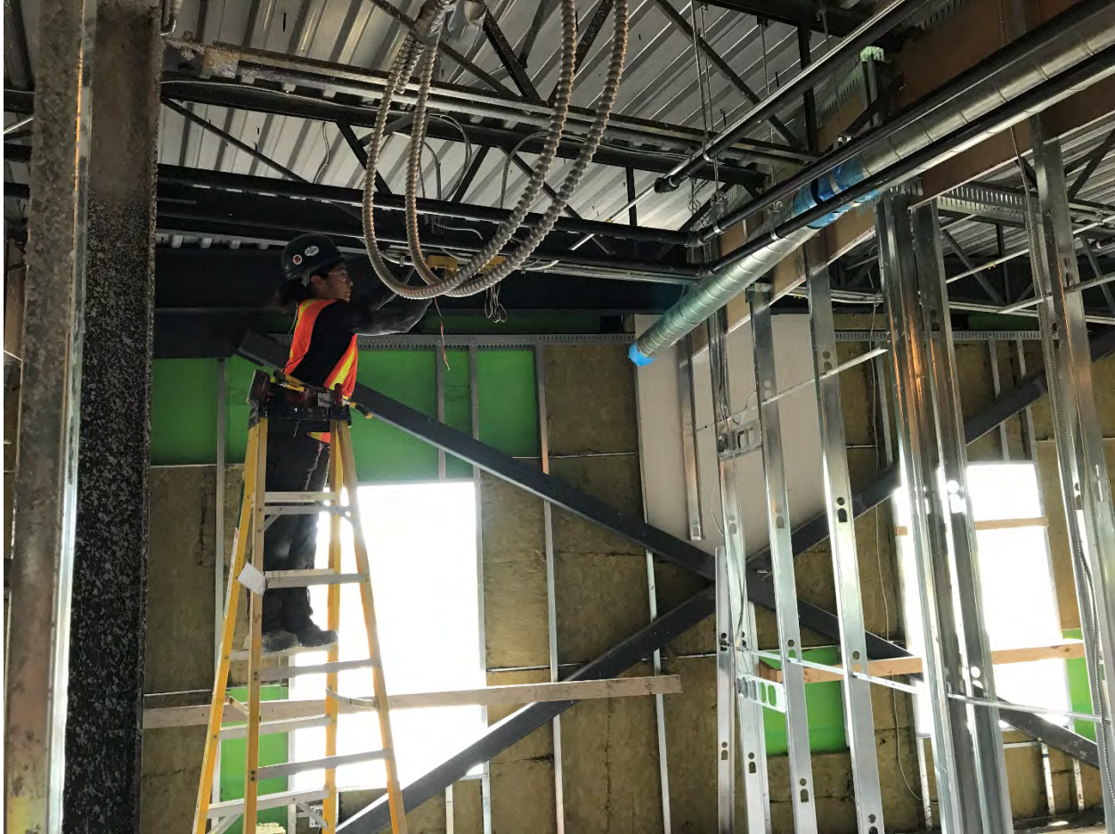
Figure 2 Example of the stage of construction on the third floor during visit on July 13, 2020.
